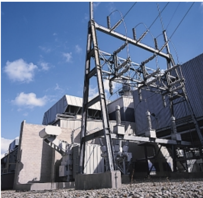
Horizon Power owns a 50-percent interest in an 80-megawatt combined-cycle natural-gas-fired power plant in North East, Pa., which it jointly acquired in April 2001. The plant provides electric power to the New York Independent System Operator, a power pool that coordinates the supply of electricity to customers in and near New York State. In addition, this plant supplies steam, a byproduct, to an adjoining grape processing plant.
