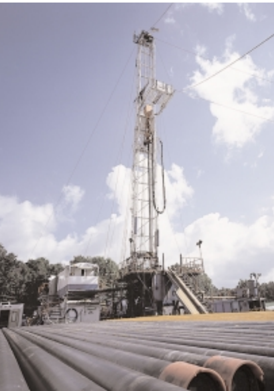
National Fuel Gas Supply Corporation's second horizontal well, at Lawtons Storage Field, has a vertical depth of 2,400 feet and a lateral length of 1,500 feet in the Whirlpool sandstone formation. This well is designed to improve the withdrawal capabilities of this field near Collins Center, N.Y.
