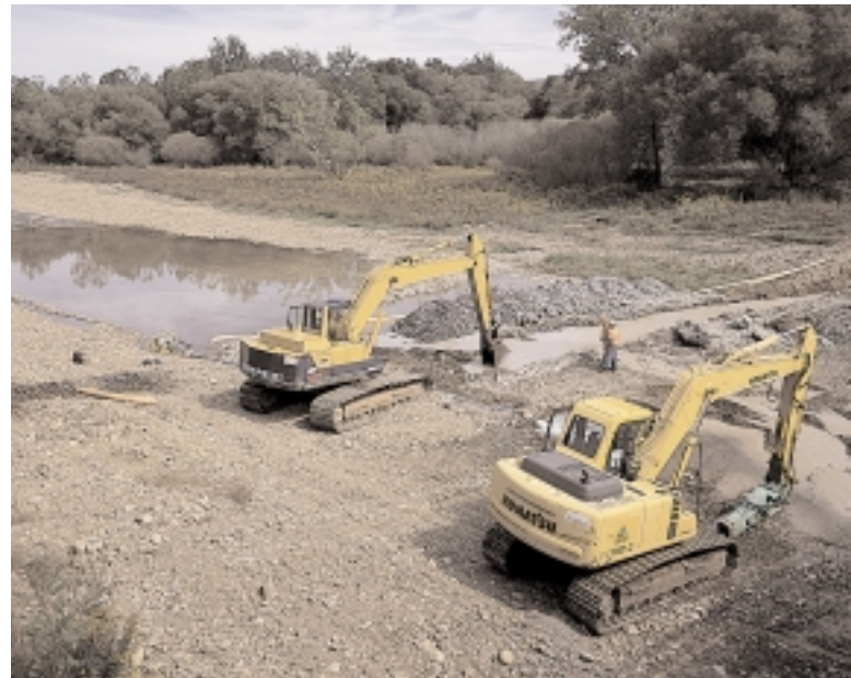
Utility crews excavated a 500-foot section of 4-inch medium pressure plastic line that crossed a 150-foot creek bed in Belmont, N.Y. after water erosion exposed the pipeline. The water was diverted around a dam during construction. One track machine broke the bedrock on the creek bottom while the other machine excavated. A 6-inch casing was set in concrete in a 3-foot trench and later, a 4-inch plastic carrier pipe was inserted into the casing.
