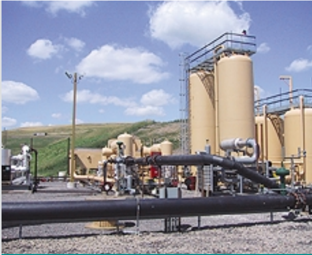
Through the acquisition of Toro Partners, National Fuel is now involved in delivering another form of energy – landfill gas. This Toro facility in Waynesburg, Ohio compresses the landfill gas, removes the unwanted components and prepares it for delivery into the Dominion East Ohio system located about nine miles away.
