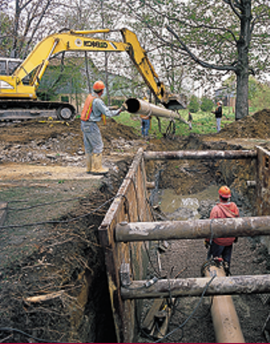
General Electric's Erie, Pa. plant, which manufactures locomotives, is in the process of replacing three coal boilers with natural gas boilers, which will produce steam for the plant. The Utility installed nearly one mile of 12-inch diameter pipeline, shown here, to meet their anticipated demand of over 300,000 cubic feet of gas per hour.
