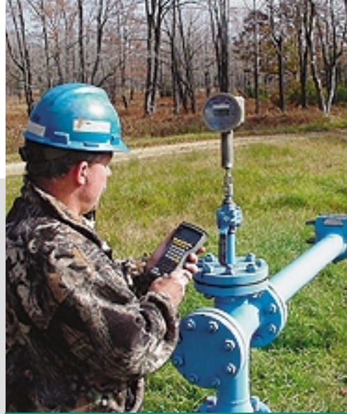
The Pennsylvania division of the Pipeline and Storage segment invested in handheld data collection technology this year to aid well tenders in electronically collecting information about its storage wells. Here, Kane Field employee Terry Johnson uses his data collector at a Wellendorf storage well near Clermont, Pa.
