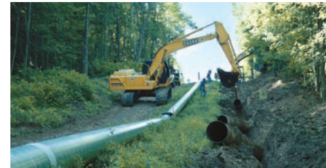
Mining activities below a six-mile section of Line N, a pipeline located outside of Pittsburgh, Pa., have caused the land around the existing pipe to sink as much as four feet, potentially compromising the pipeline's structural integrity. To ensure Line N's future safety and reliability, a new pipeline will be constructed parallel to the 57-year-old line.*
