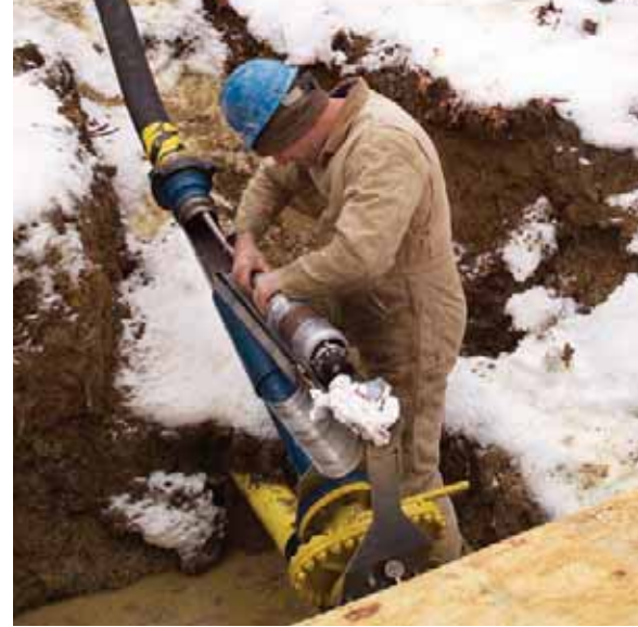
A National Fuel employee prepares to evaluate a four-inch pipeline at the Company's Colden Storage Field.
