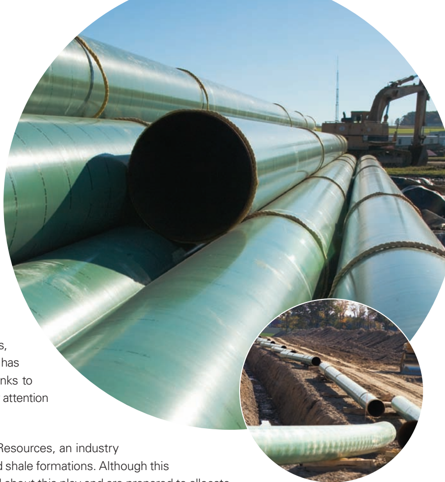
In September, construction began on the 78-mile-long Empire Connector Pipeline Project. Phase One involved approximately 19 miles of the 24-inch pipeline (shown here) to be installed in Yates and Schuyler counties. Phase Two will commence in spring 2008, with the remaining mileage to be completed by November.
