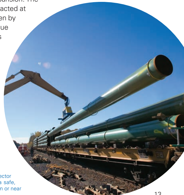
80-foot sections of the Empire Connector Pipeline are removed from rail cars arriving from Louisiana, where our custom-ordered pipe was manufactured.
