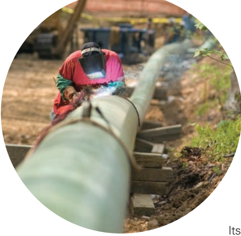
A welder works on a pipeline replacement project in Allegany State Park's popular Thunder Rocks area. Known for its primitive forested valleys, un-glaciated landscape, fall leaves and wildlife, this park has been home to our pipeline for decades where it has co-existed with this natural treasure without incident or intrusion.
