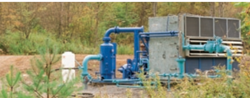
The R-49 compressor pictured above was installed in 2009 to help bring local gas production from existing wells owned by Seneca and third-party producers to market.
