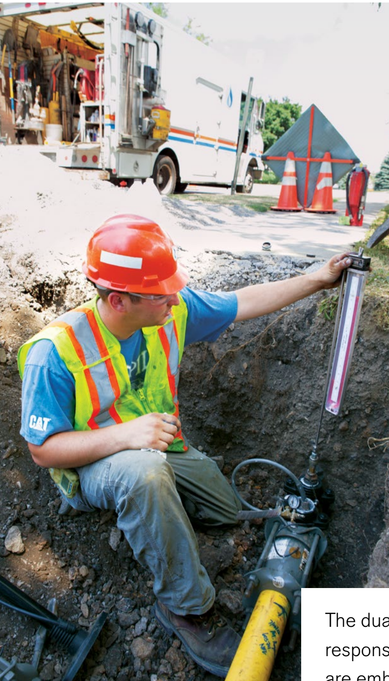
▲ Michael Argauer of the Company's Utility subsidiary inspects a low-pressure distribution line in Lackawanna, N.Y., maintaining National Fuel's commitment to operating a safe and reliable system.
