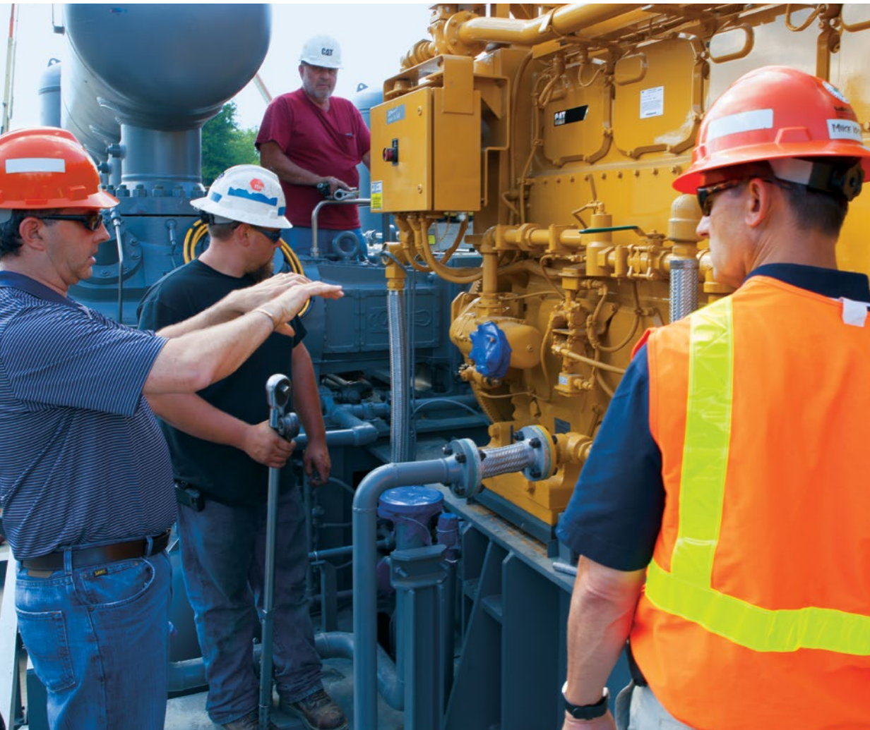
▼ Terry Kreuz and Mike Kasprzak of National Fuel Gas Supply Corporation monitor construction progress on the Northern Access Expansion Project that transports natural gas to Canadian markets.
