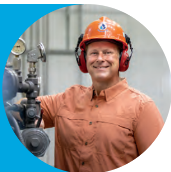
Supply employee inspects an upgraded compressor unit in Mercer County, PA. New unit equipment helps to improve efficiency and lower emissions.
