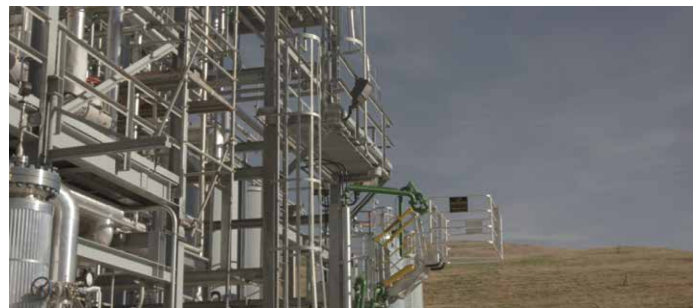
From landfill gas to product offtake (foreground).
