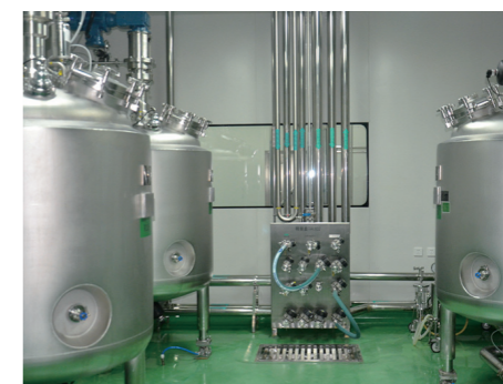
S/D Inactivated Heat Preservation Tank
