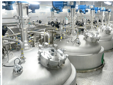
Closed Reaction Tanks
