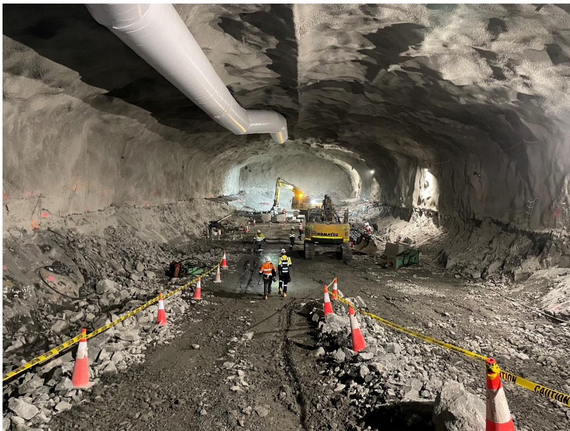
Above: Underground Power Station Cavern, 250MW Kidston Pumped Storage Hydro Project, North Queensland
