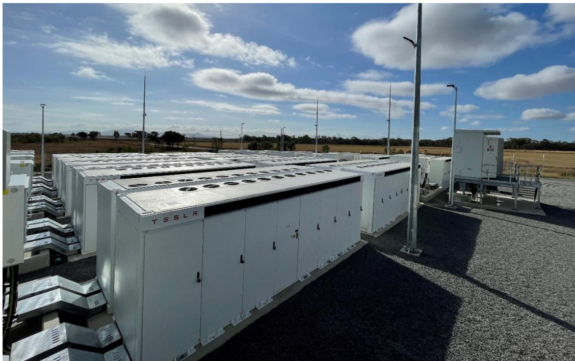
Above: 50MW/100MWh Bouldercombe Battery Project, Central Queensland
