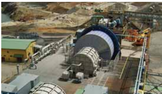
Mill SAG – Process plant at Cerro Corona
