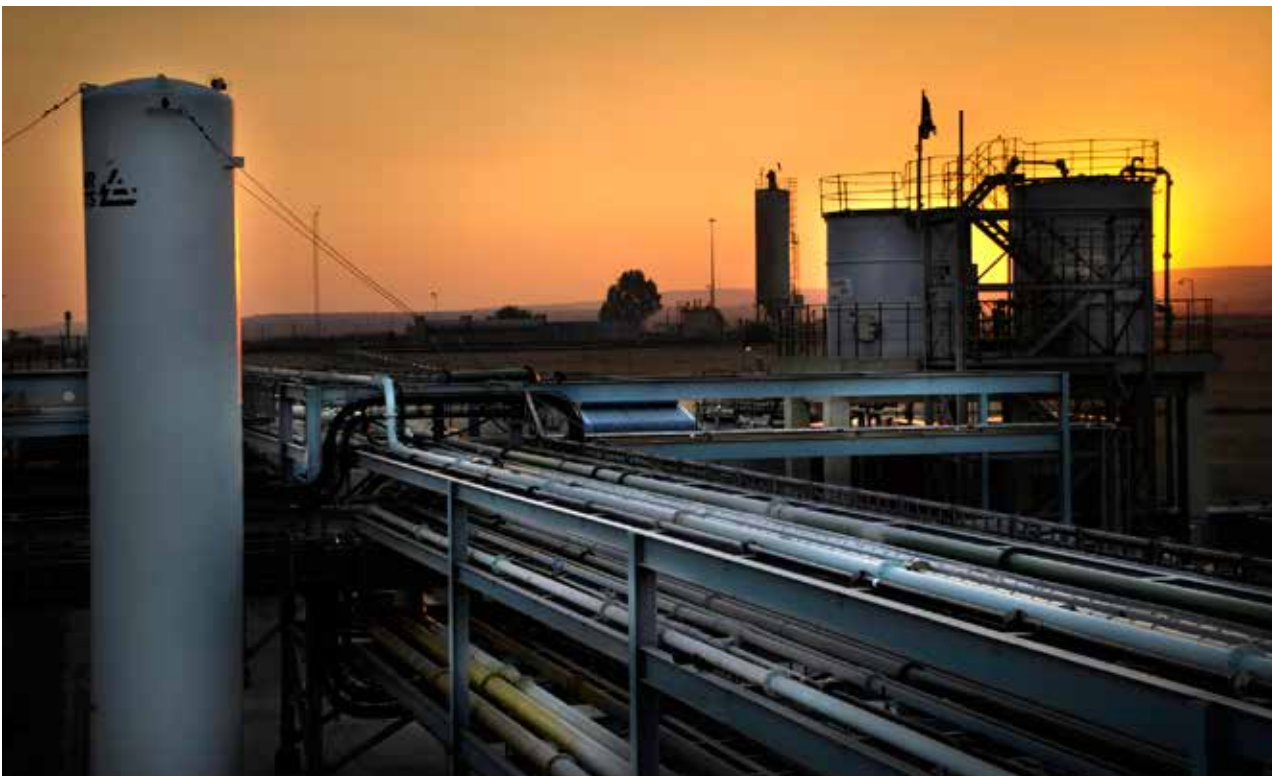
› South Deep plant
