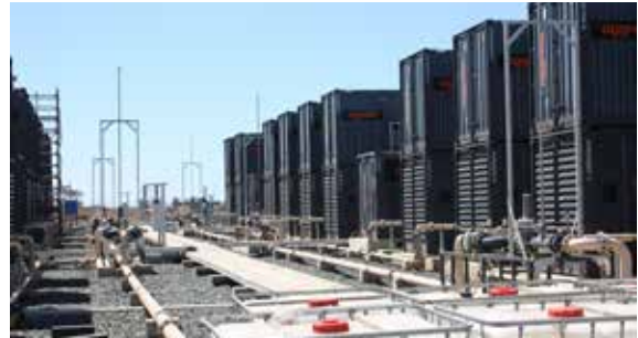
Granny Smith gas plant
