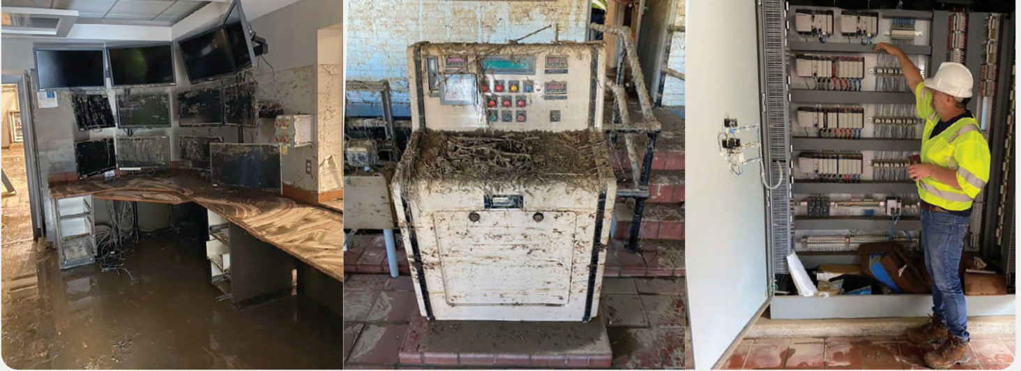
Damage sustained at Pickering West Water Treatment Plant during Hurricane Ida.
