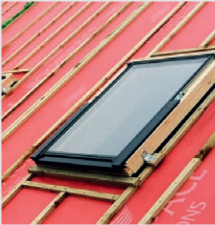
Closed panel roof systems installed at our sites at Beechwood in the North East, above, and Kibworth Green in the North Midlands, below.
