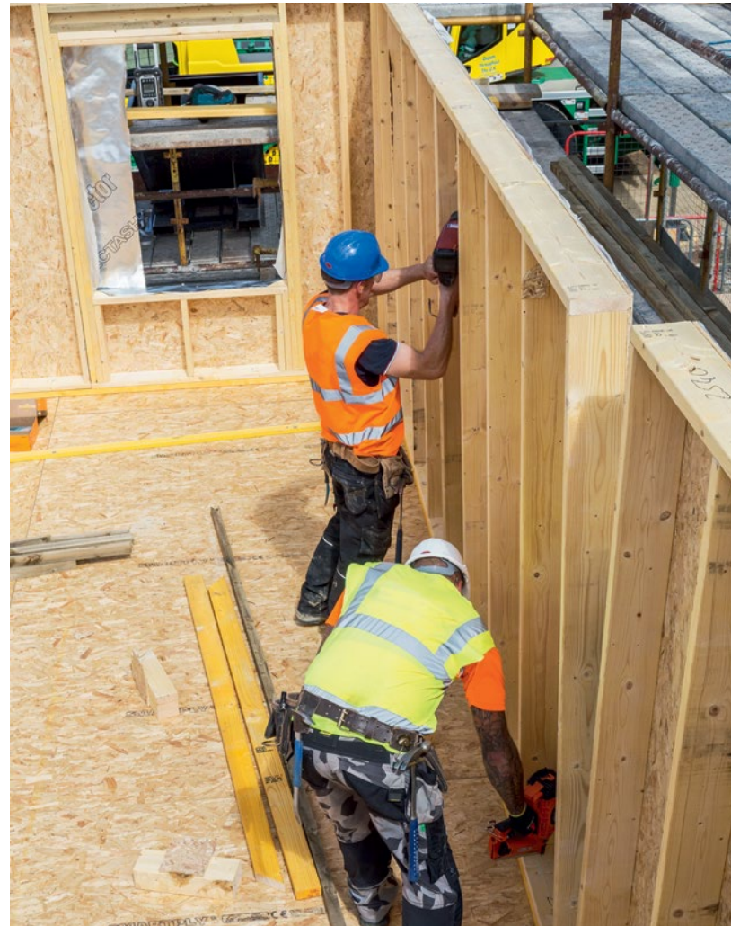
Timber frame external wall panels being fixed into place at our Osprey Heights development in Inverurie, Aberdeenshire.
