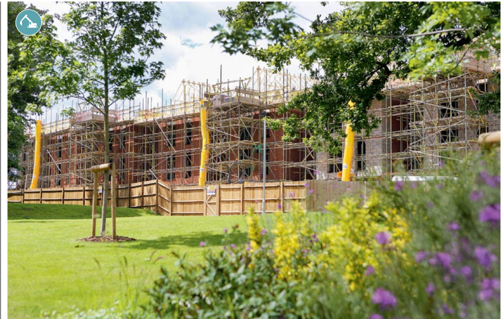
Cane Hill Park in Coulsdon, Surrey where we are trialling the use of Light Gauge Steel Frames in the construction of apartments and using timber frames in the construction of houses.
