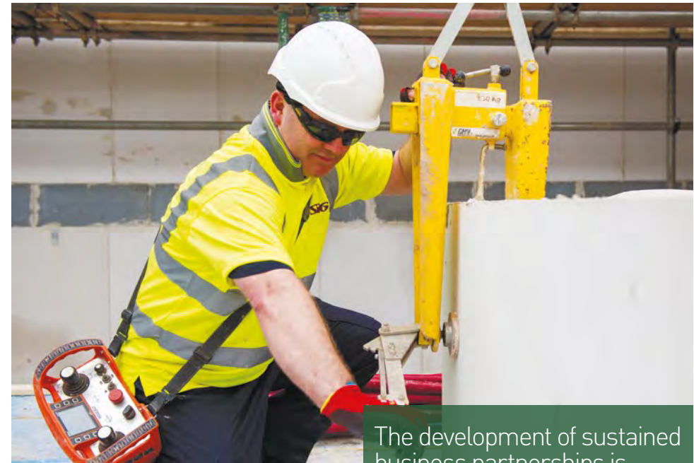
A crane driver from our partner SIG Roofspace Ltd attaching the clamp to the Large Format Block in readiness for lifting.
