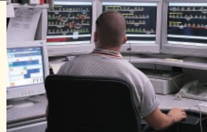
Above: The NY/PA state-of-the-art dispatch system is a "point and click" system with the railroad operating rules written into the computer program. This allows dispatchers to save time, eliminate errors and control movement on the track more safely.
