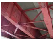
A bridge beam (in its 16 th year) without LUMIFLON coating
