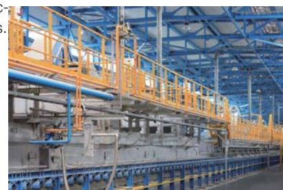
One of the world's largest glass production facilities, which came on line at the Klin plant in Russia
