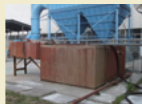
Tank for wastewater reuse
