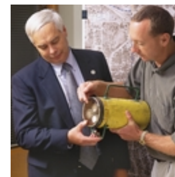
Jim Morgan (left), Madison's superintendent of parks, and Craig Fenrick, MGE executive director — electric transmission and distribution, examine underground cable for new electric facilities in Madison.
