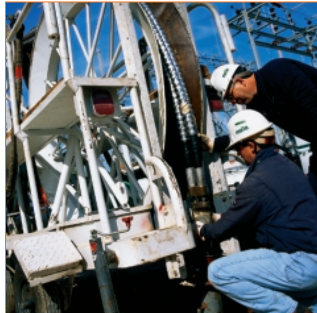
MGE installed a large underground transmission line to bolster reliability on Madison's west side. MGE employees Bart Schley (left), Line and Cable Technician, and Dale Barnes, Line Technician, helped install six miles of electric cable to energize a new substation. Advance planning with local and state agencies, elected officials and area residents ensured timely construction of this vital project. American Transmission Company owns and operates the line.
