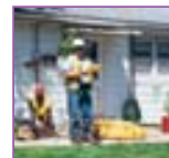
MGE finished a three-year project in Prairie du Chien, replacing all copper services with plastic pipes. MGE Distribution Fitter LuWayne Mathson (standing) checks on the progress of work at a
