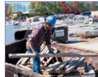
MGE recycled enough waste wood, cardboard and paper to save nearly 1,900 trees so far while building the West Campus Cogeneration Facility. About 1,500 tons of concrete and metal also were recovered and reused. With help from WasteCap Wisconsin, Inc., 85% of the construction waste was recycled, surpassing MGE's goal.
