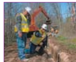
Key gas system projects help meet growing demand – from Madison's east side to western Dane County. MGE Foreman Francis Stanek (left) and Steve Stehling, MGE Manager – Gas Systems Engineering, inspect a new gas main that increases pressure and reliability for fast-growing Mt. Horeb and communities to the west.
