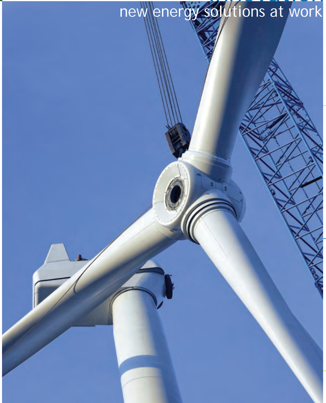
At MGE Energy's new wind farm, a crane hoists the blades to the top of a 260-foot-tall tower.
