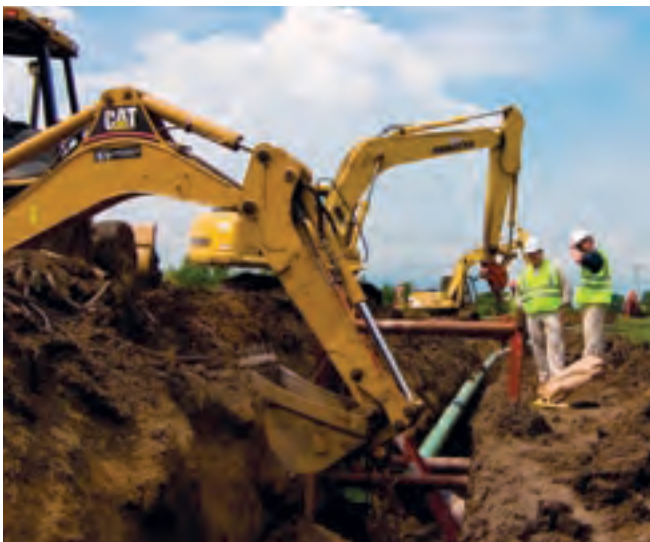
Steve Beversdorf (left) and John Wichern, MGE gas systems engineering technicians, check the progress of a gas construction project on Madison's growing west side.
