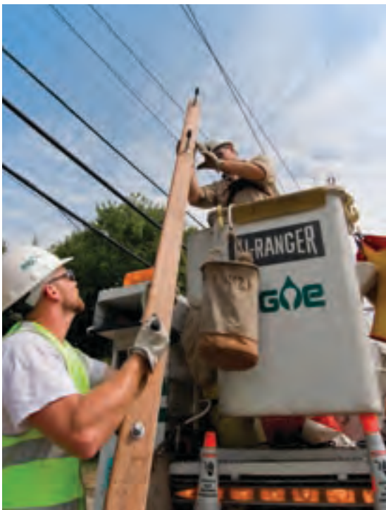
Regular maintenance is critical for a reliable electric system. Rob Priestley (left) and Bob Harper, MGE line technicians, replace a cross arm on a power pole.
