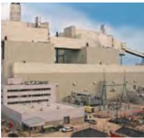
Construction at the Oak Creek Power Plant, located on Lake Michigan, began in June of 2005 and will wrap up later in 2010.
