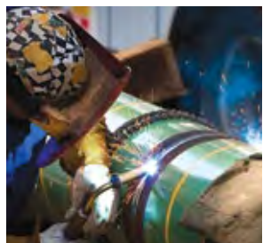
Brad Gordon, an MGE pipe-fitter, welds a steel gas main during a recent project.
