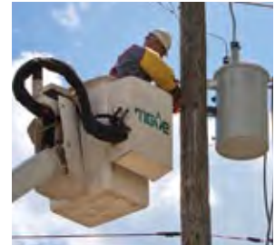
Troy Shawback, an MGE line technician journeyman, works on a transformer. MGE puts a priority on maintaining its electric distribution system.
