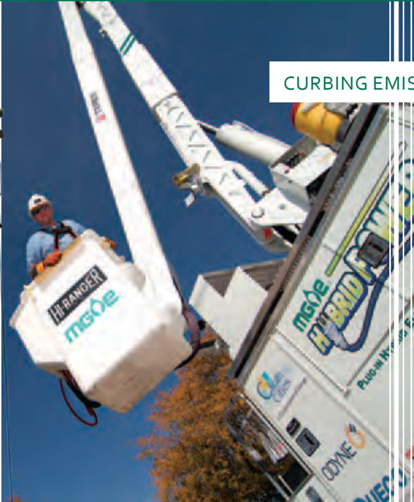
Nate Berg, an MGE line technician, operates a hybrid bucket truck. The hybrid component operates the aerial lift rather than depending on an idling truck engine.
