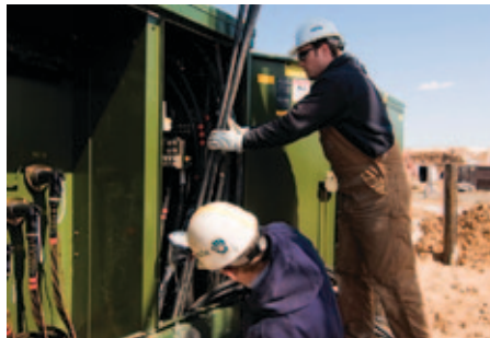
An MGE electric crew pulls cable that serves the TEAM Companies data center.
