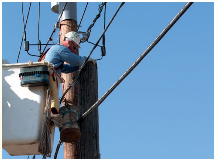
Josh Shepard, an MGE crew leader, works on the distribution system near downtown Madison. Upgrades of the electric system help maintain high reliability.
