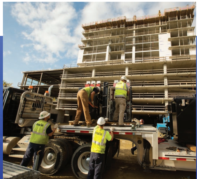
MGE crews unload a large electric transformer to help power a new high-rise development with 244 apartments. Madison's East Washington Avenue is a growing hot spot for high-end housing and commercial space.
