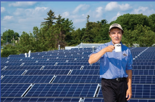
Mark Ballering, owner and founder of Steep & Brew Coffee, installed an 80-kilowatt photovoltaic system atop the roof of his office, roasting facility and distribution center.
