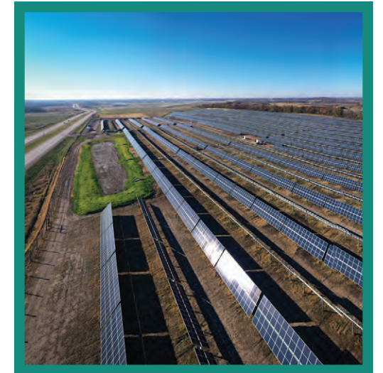
In December, MGE's 9-megawatt solar array at the Dane County Regional Airport came online. The project, visible from Highway 51, serves Dane County operations, advancing both MGE's and the County's sustainability goals.
