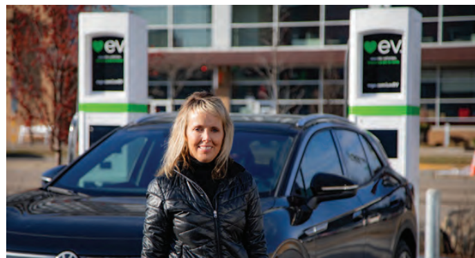
MGE’s new EV fast-charging hub, powered by renewable energy, features some of the most powerful chargers in the region. MGE Manager of Electrification Debbie Branson says adding fast-charging infrastructure is key to getting more EVs on the road.
