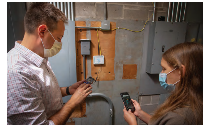
MGE Senior Account Manager in Commercial and Industrial Marketing Matthew Matenaer shows Dane County Director of Facilities and Services Amanda DePogter how new submetering technology will help the County more accurately track and manage energy consumption at the Dane County Job Center in Madison.
