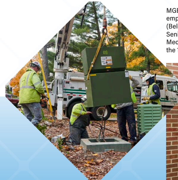
MGE's distribution system is evolving with our grid and our community. In addition to investing in renewable resources, MGE is working to upgrade its distribution system through our grid modernization projects to bring enhanced reliability and grid monitoring and control technologies to better serve customers.
