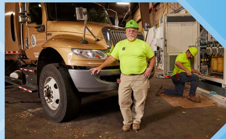
Matt Parks (foreground), Master Electrician, and Mathias Kranz, Journeyman Electrician, both with the City of Madison Engineering Division, finish installation of a charging station provided by MGE to power the City's first electric refuse trucks, expected in 2024.
