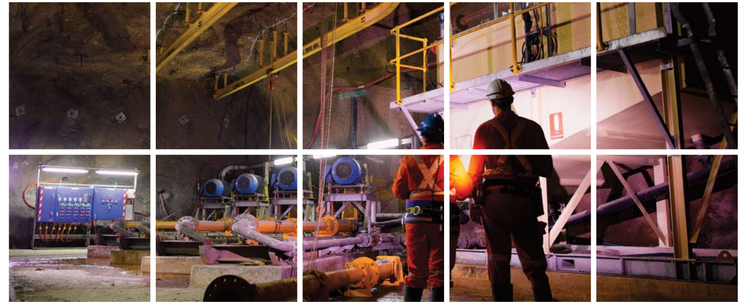
Above: Pumping station, Gwalia underground Right: Processing plant, Leonora
