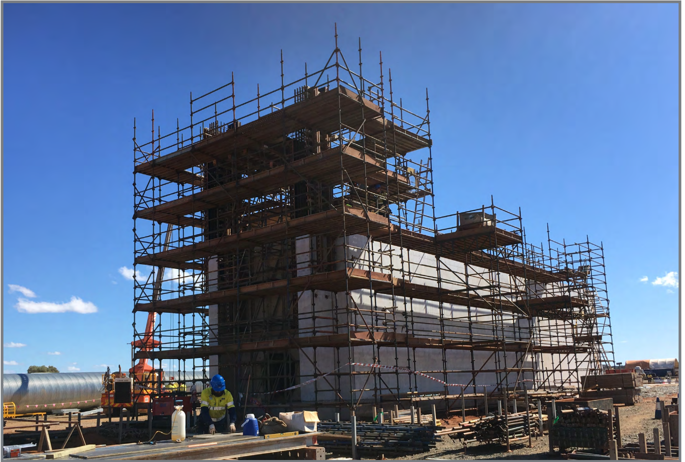
Figure 4: - Construction of the Transfer Vault that will lie beneath the Coarse Ore Stockpile (refer Figure 3).
