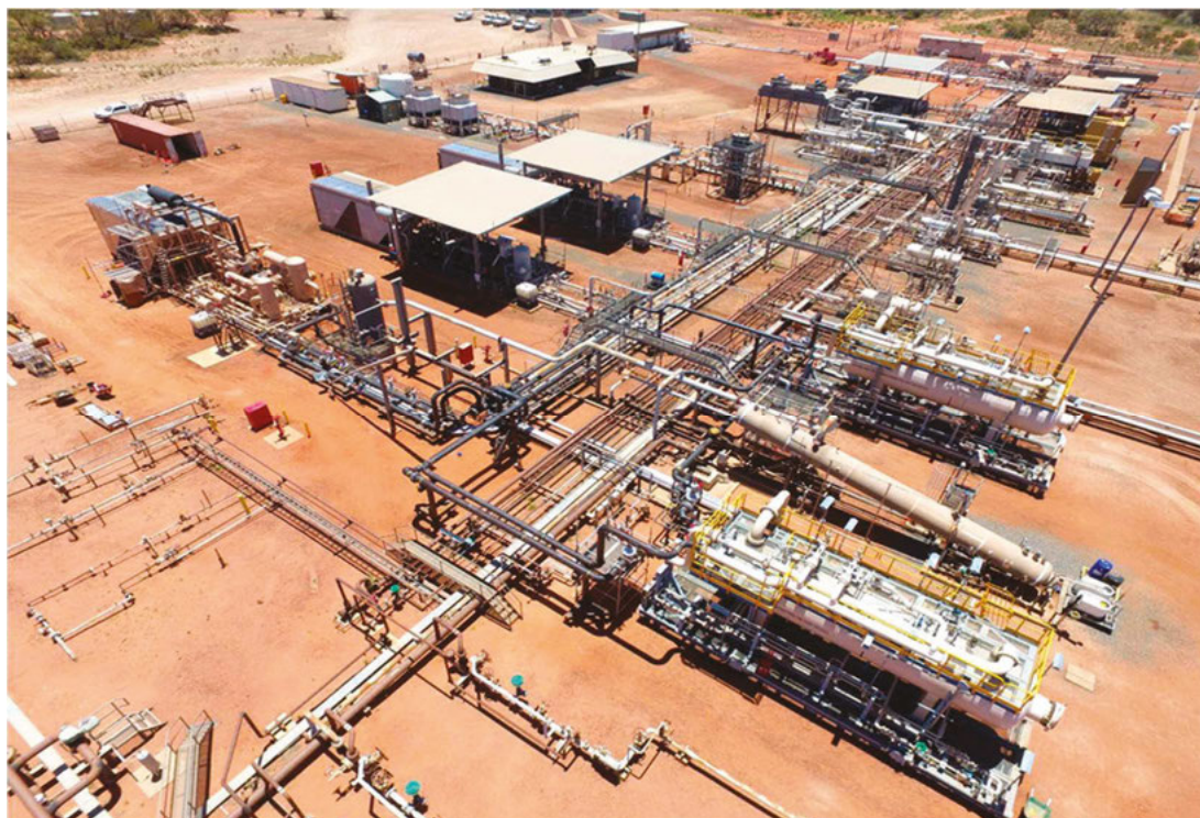
New equipment installed as part of the Mereenie Facility Upgrade
