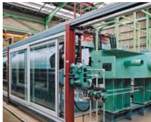
Membrane-process chlor-alkali plant
