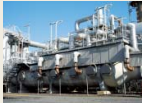
Equipment for thermal decomposition of N 2 O
