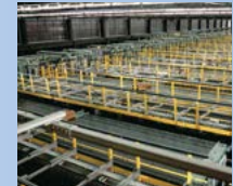
Membrane-process ion-exchange plant
