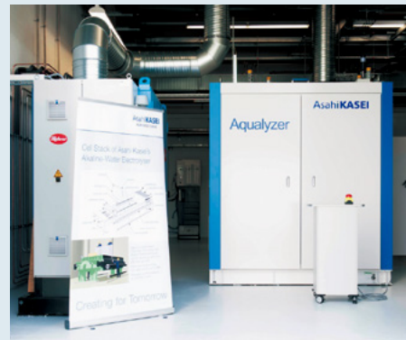
The demonstration plant in Herten, Germany
