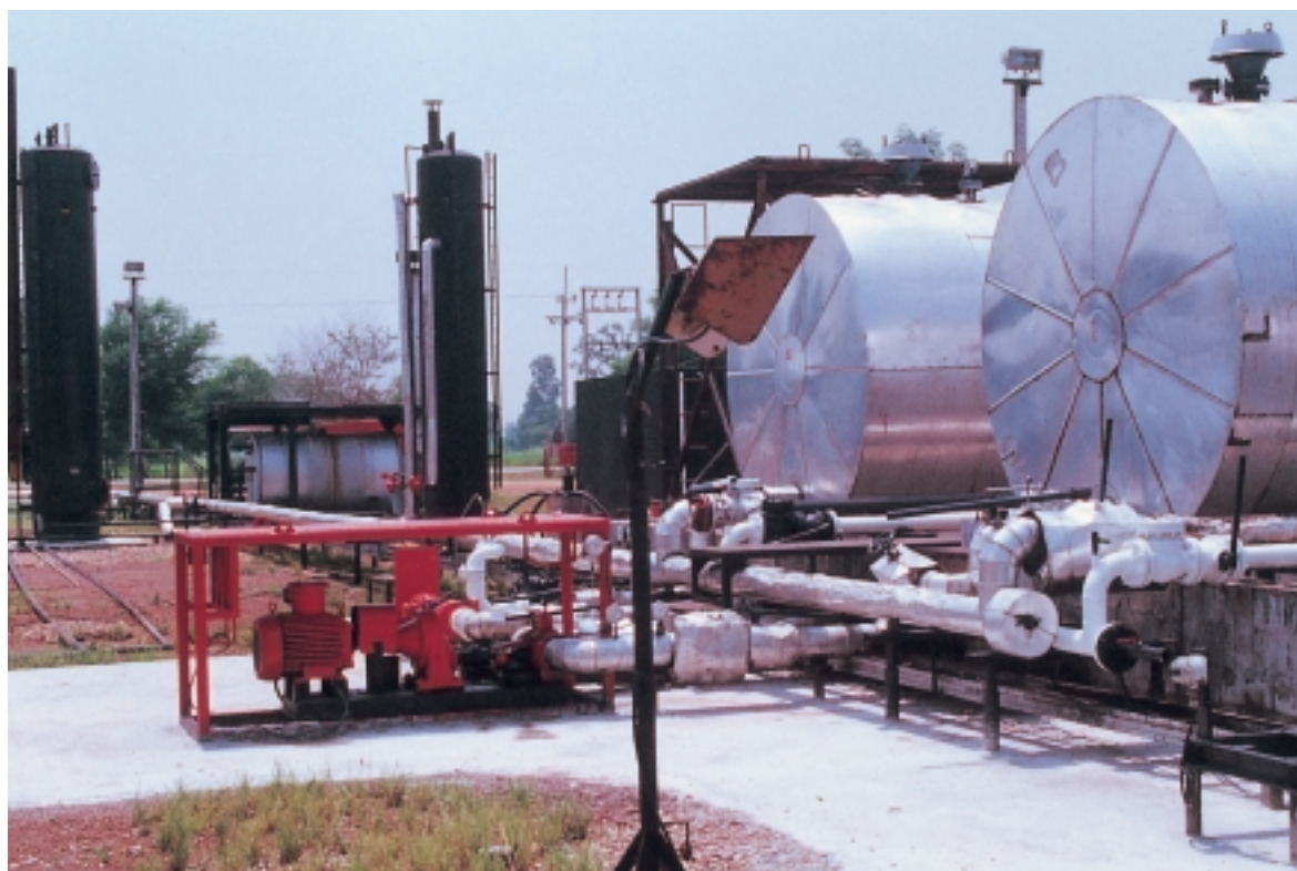
Production facility adjacent to WB-1 well, SWIA Concession, Central Thailand.
