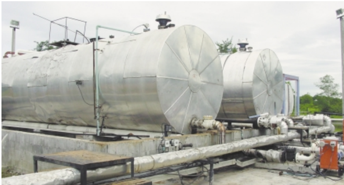
Production storage tanks, WB-1, Thailand
