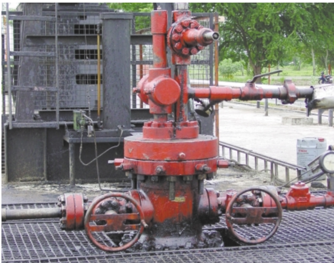
Well head at WB-1, Thailand
