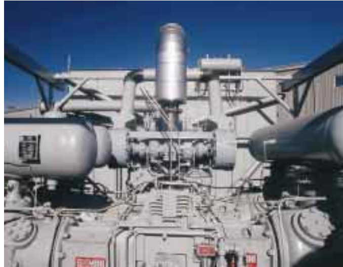
A skid mounted portable natural gas compressor.
