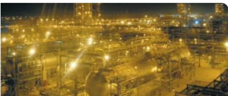
Khurais Crude Facilities, Saudi Arabia
