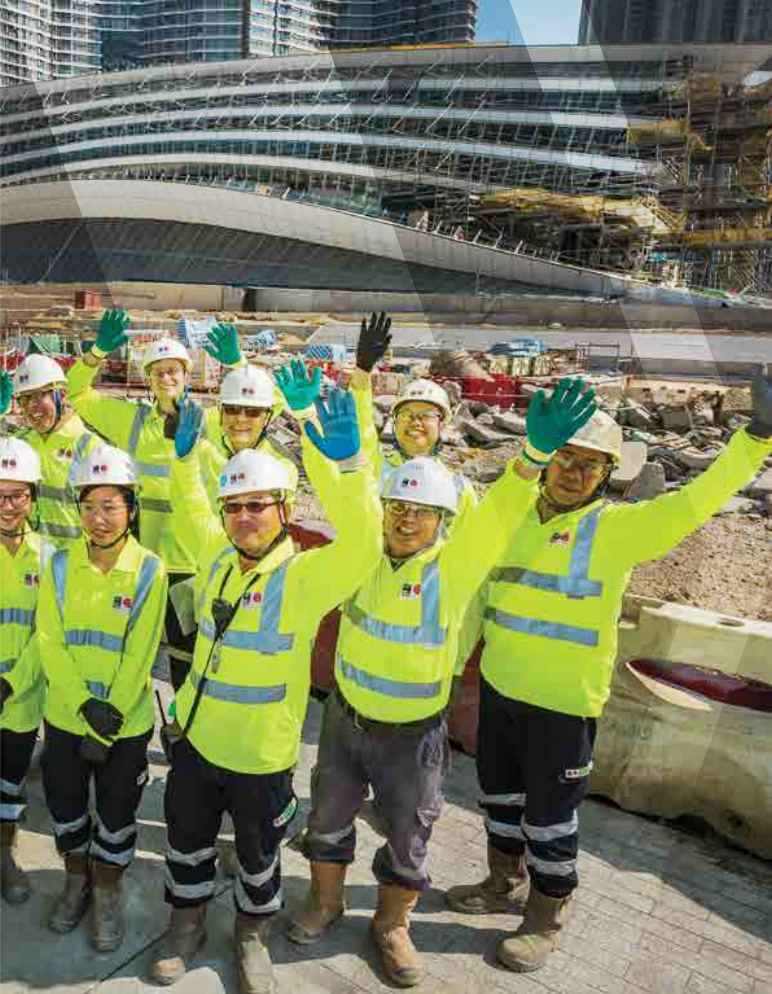
Photo: Express Rail Link, West Kowloon Terminus Station North project, Hong Kong, Leighton Asia.
