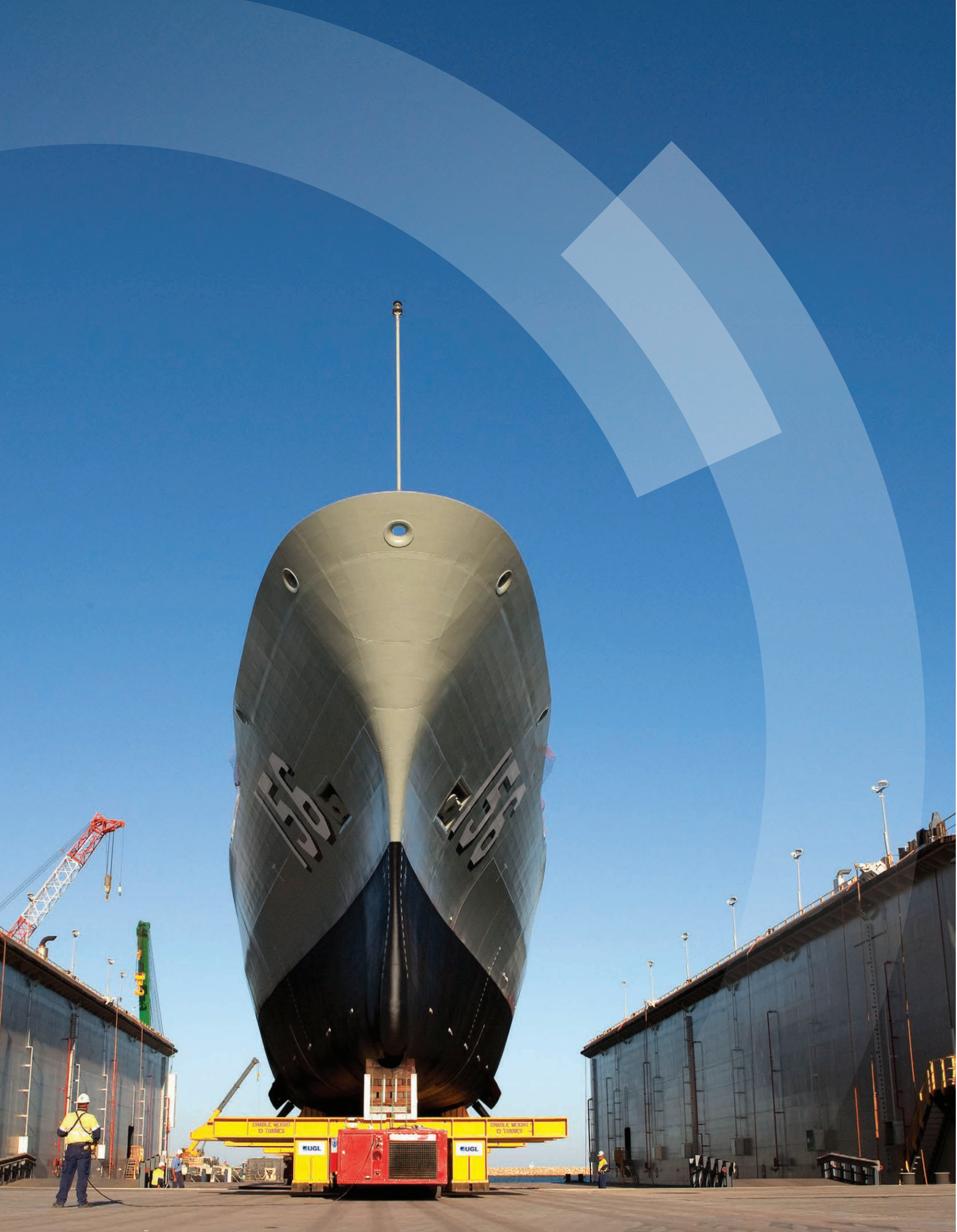
Maintenance Docking of HMAS Toowoomba, Henderson Common User Facility UGL, Western Australia
