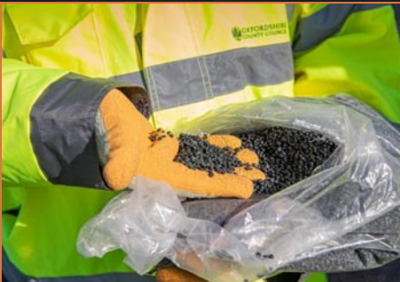
Above: A picture taken during the resurfacing of a 700-metre stretch of Marsh Lane in Oxford that will be laid with Gipave ® , a graphene-enhanced supermodifier for asphalt pavements, with the rest resurfaced using conventional asphalt, so that the two can be accurately compared. Above right: Graphene nanoplatelets.
